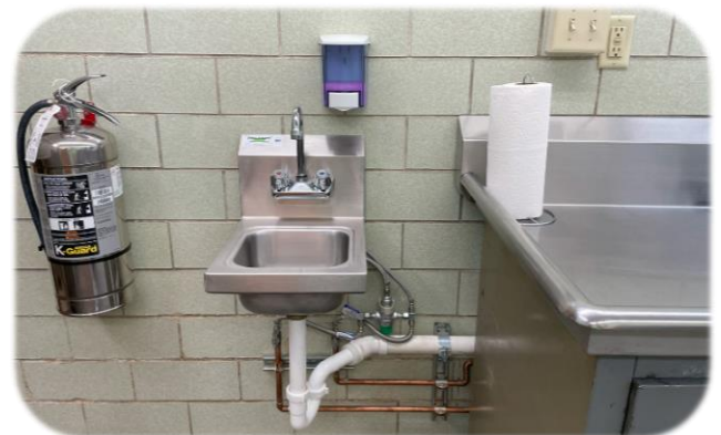
New hand washing sink
